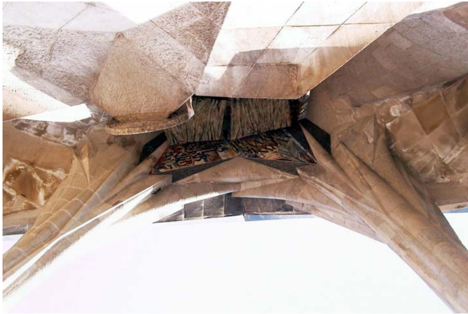
Fig 8. Hyperbolic paraboloid 'branches' overlapping and meeting on their directrices in the Passion Façade
